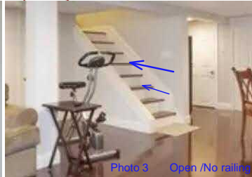
Photo 3 Open /No railing
